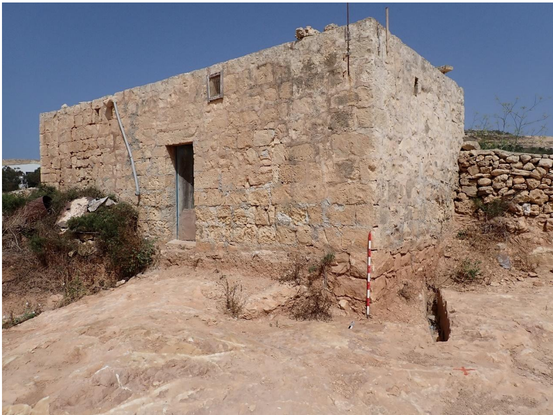
FIGURE 51: DILAPIDATED FARMHOUSE IN THE NORTHERN PART OF SITE, LOOKING NORTH
