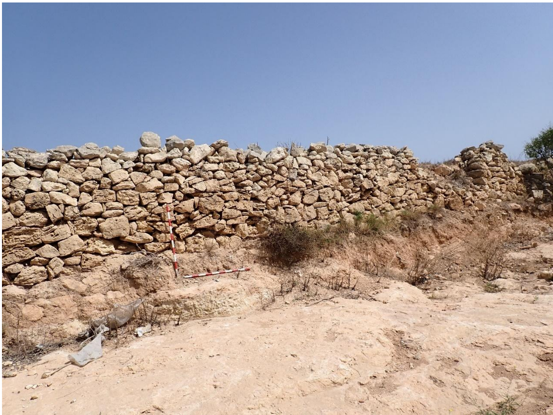
FIGURE 57: NORTHERN RUBBLE BOUNDARY WALL IN POOR CONDITIONS, LOOKING NORTH
