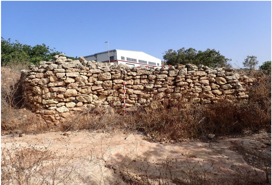
FIGURE 10: WESTERN ACCESS TO SITE, RUBBLE BOUNDARY WALL BETWEEN SITE AND WASTESEV TREATMENT FACILITIES, LOOKING NORTH
