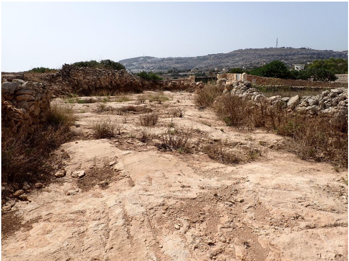
FIGURE 45: RUBBLE BOUNDARY WALLS IN POOR CONDITION IN THE SOUTHERN ACCESS TO SITE, LOOKING SOUTH
