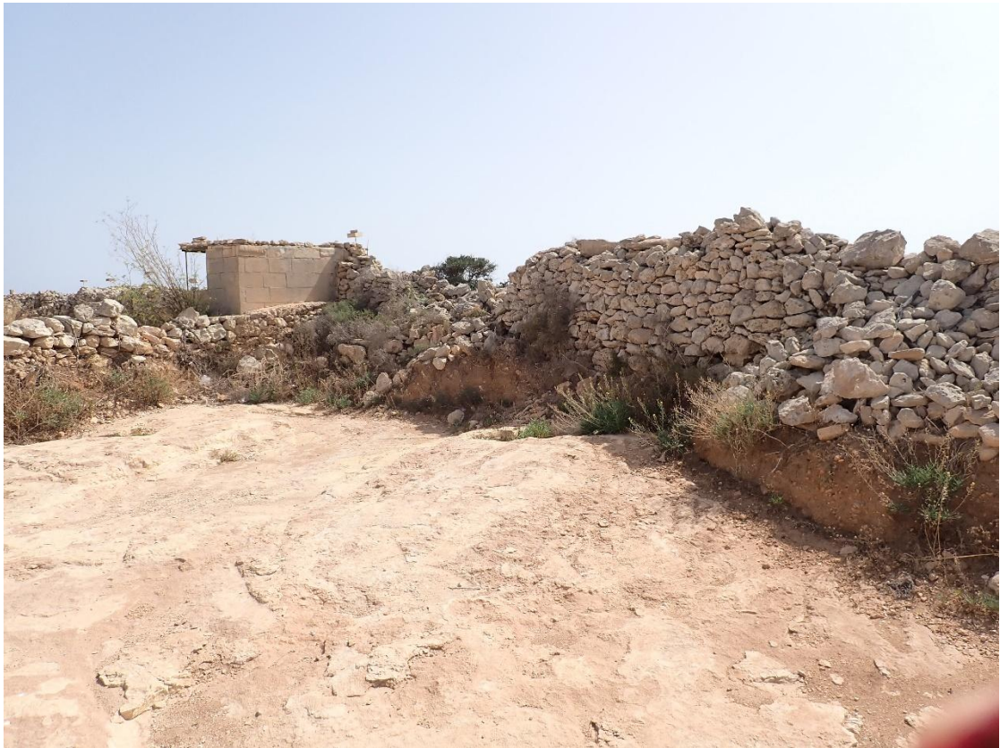
FIGURE 46: RUBBLE BOUNDARY WALLS IN POOR CONDITION IN THE EASTERN PART OF SITE, LOOKING SOUTH
