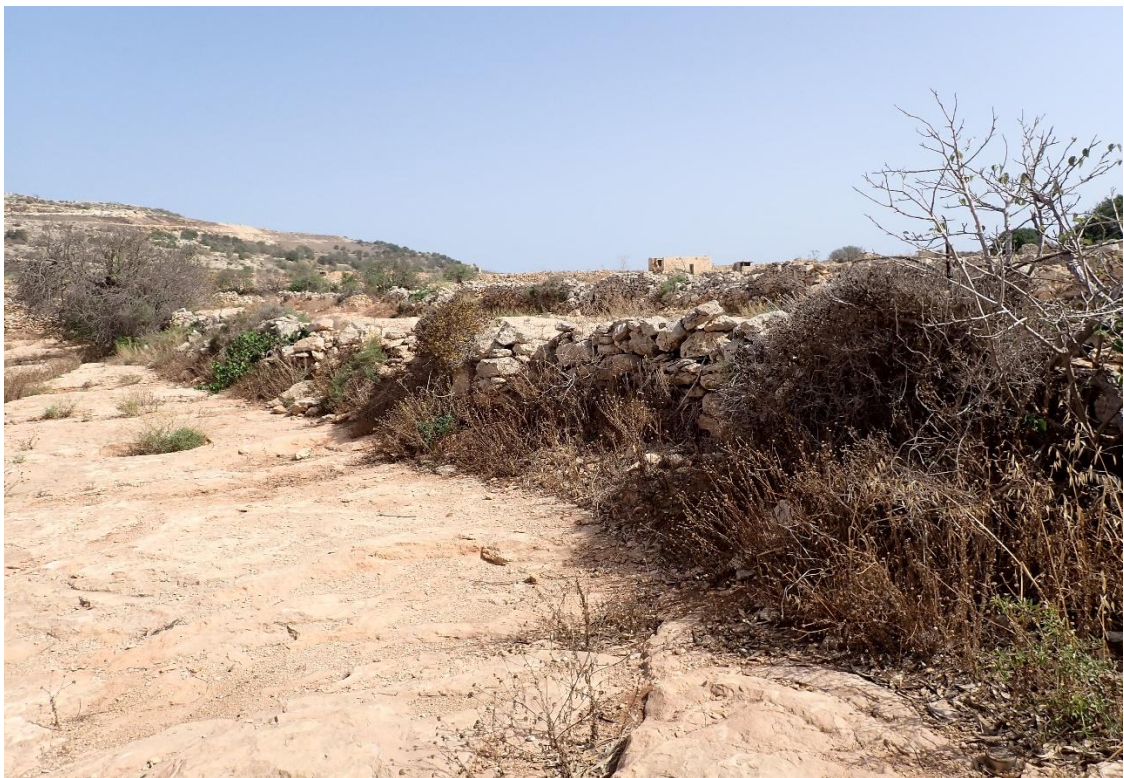
FIGURE 43: RUBBLE BOUNDARY WALL IN POOR CONDITION IN THE EASTERN AREA OF SITE, LOOKING N-EAST
