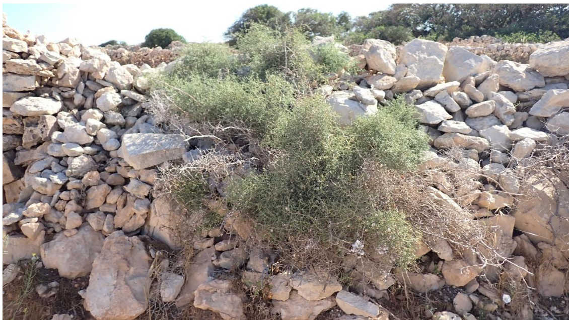
FIGURE 25: VEGETATION GROWING WITHIN DEGRADED RUBBLE WALLS AND RUBBLE STRUCTURES (PHOTO TAKEN JULY 2024)
