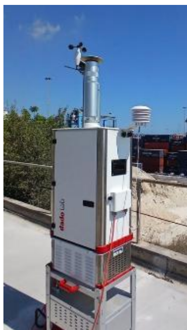
FIGURE 20: SEQUENTIAL AUTOMATIC SAMPLER INSTALLED ON SITE
