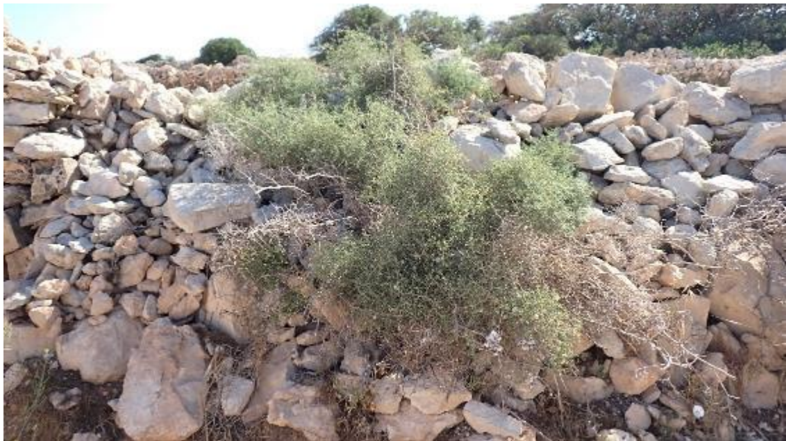
FIGURE 26: VEGETATION GROWING WITHIN DEGRADED RUBBLE WALLS AND RUBBLE STRUCTURES (PHOTO TAKEN JULY 2024)
