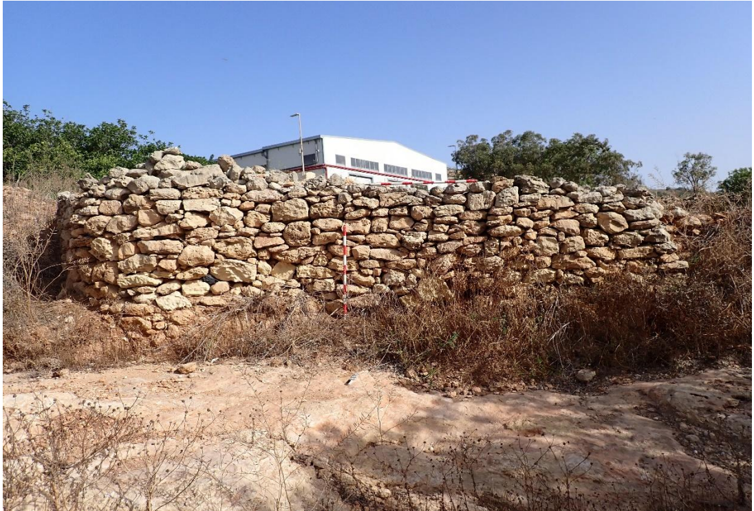
FIGURE 101: WESTERN ACCESS TO SITE, RUBBLE BOUNDARY WALL BETWEEN SITE AND WASTESEV TREATMENT FACILITIES, LOOKING NORTH
