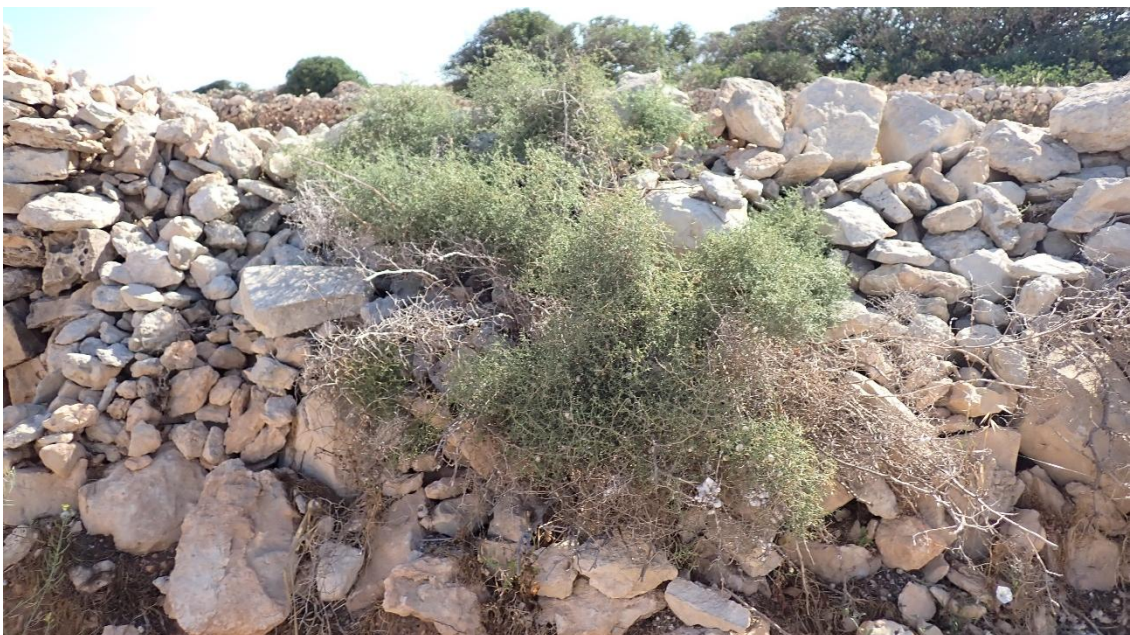
FIGURE 82: VEGETATION GROWING WITHIN DEGRADED RUBBLE WALLS AND RUBBLE STRUCTURES (PHOTO TAKEN JULY 2024)
